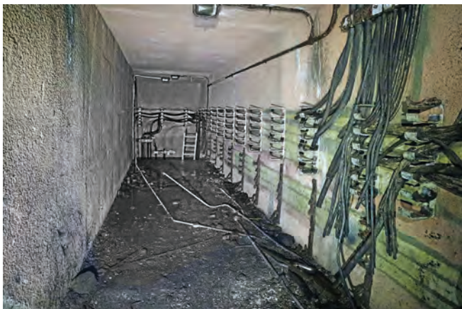
The high level emergency exit tunnel. The emergency exit is behind the photographer. Note the ladder at the far end which leads down to the bunker. The stairs here were removed by contractors before the bunker was sold
